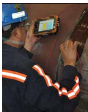
QUALITY CONTROL Once the welding is complete, the can is visually inspected by Quality Control (QC) and, if required, Ultrasonic (UT) testing is performed to ensure the weld is defect-free.
