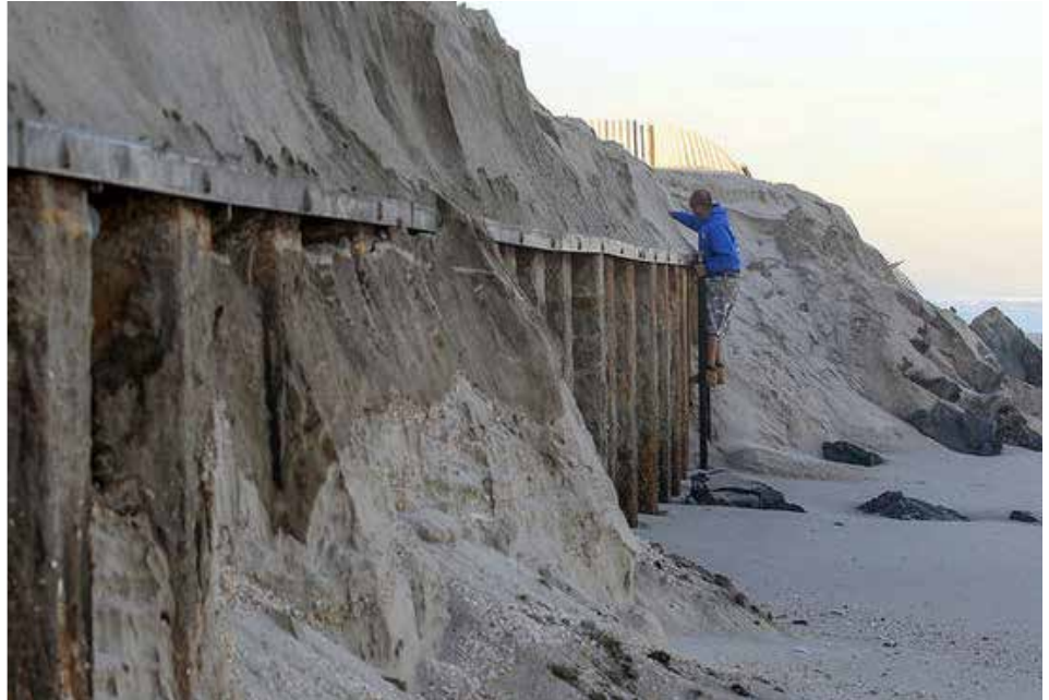
A man uses an emergency escape ladder to get off the beach in Mantoloking after climbing down to the ocean's edge east of the massive steel wall - which is now exposed - a barrier that is providing a last line of defense. (PHOTO: Andrew Mills | NJ Advance)
