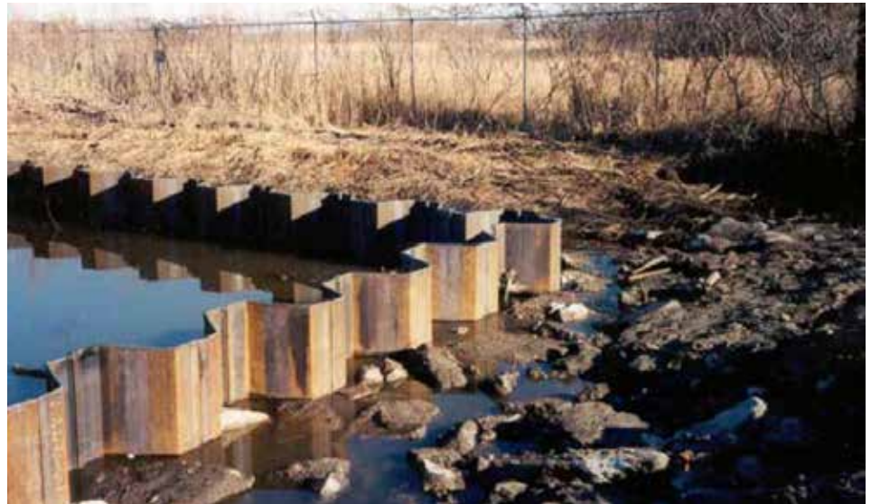
Above: Two walls of the cofferdam meeting before the closure piles were placed. Since good closure of the cofferdam was necessary the T-connection was fabricated on site.
