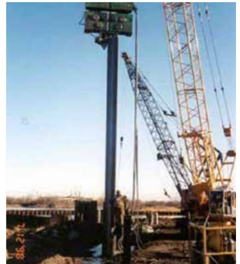
Water elevation difference, about four feet, between the inside of the cofferdam, (to the left of the wall on the left), and the outside of the cofferdam, (between the two rows of sheets and to the right of the outer wall). The outer wall was an old wall which had no sealant.
